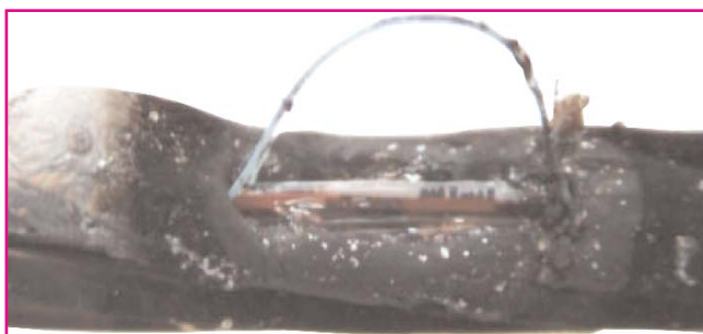
The extensive damage caused by a lightning strike on steel cable. The fibre is exposed and the cable requires replacement.
